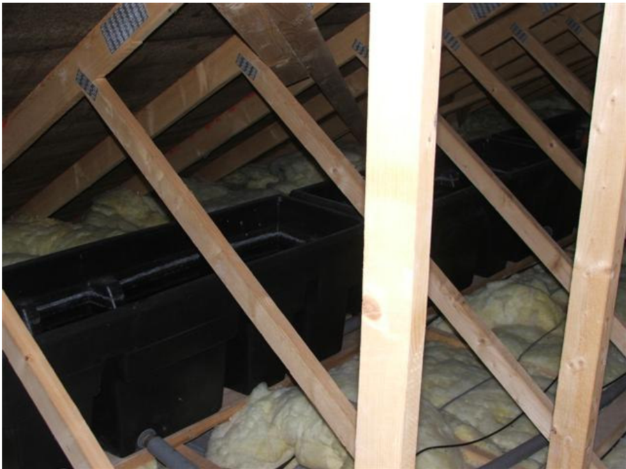
Photo 8: Showing the water tank uninsulated.
