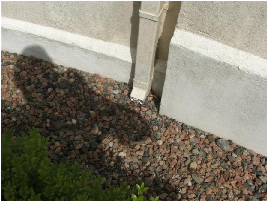
Photo 5: Showing no surface water gully trap.
