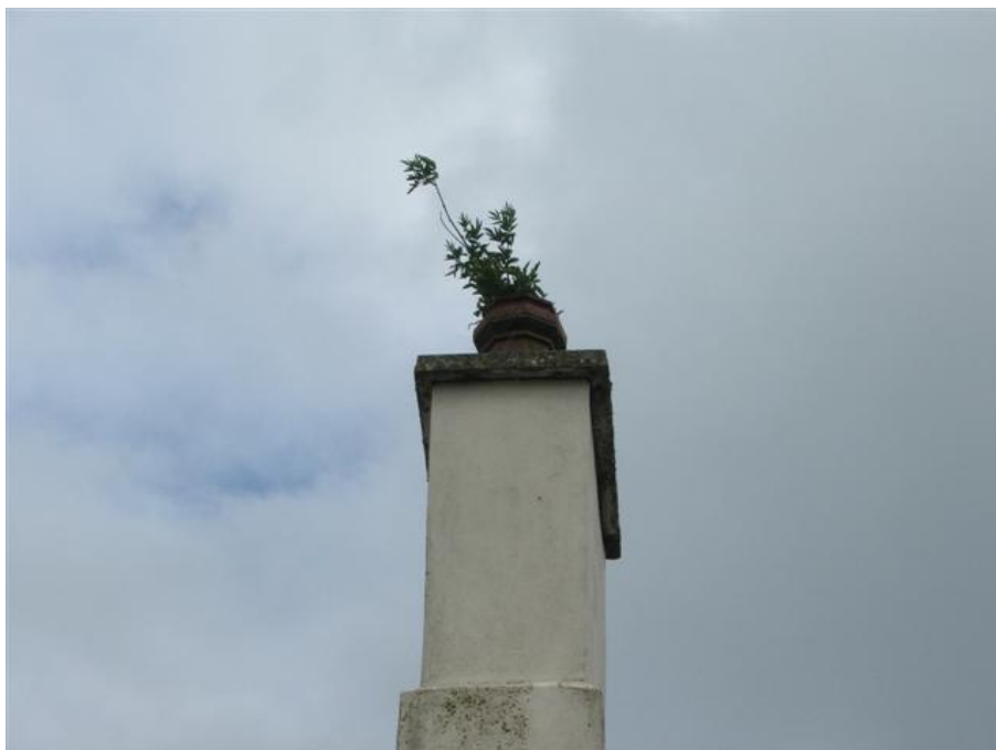
Photo 2: Showing vegetation in chimney.
