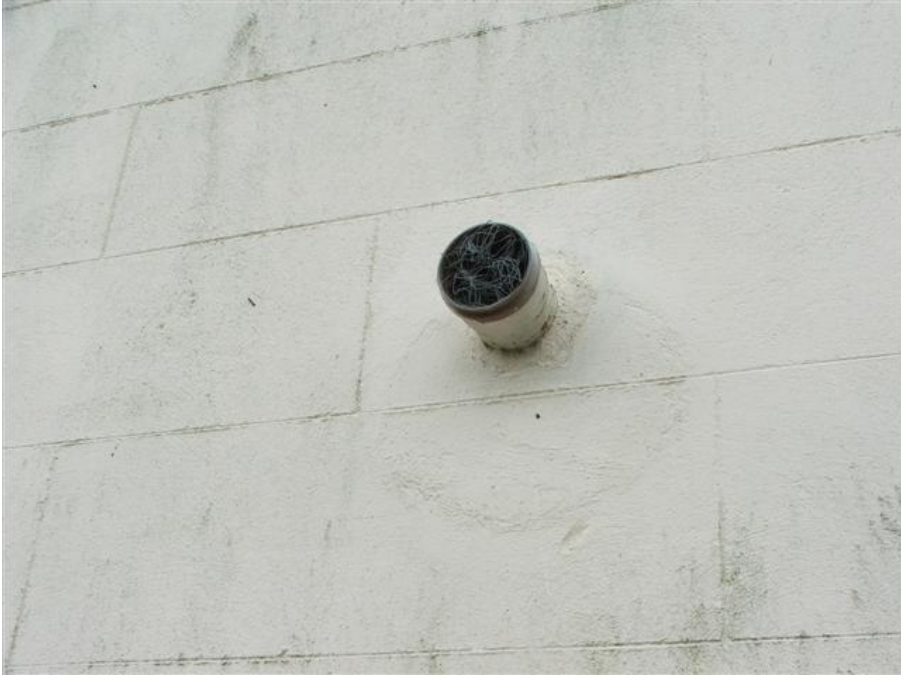
Photo 3: Showing poor finish to extract vent from kitchen.
