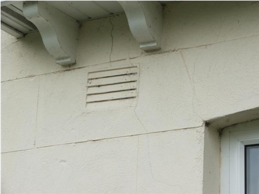
Photo 4: Showing expansion crack to wall.
