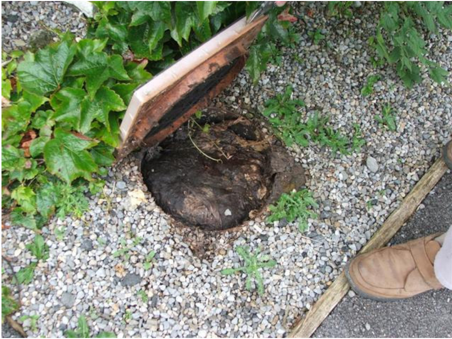
Photo 7: Showing the blocked foul sewer.
