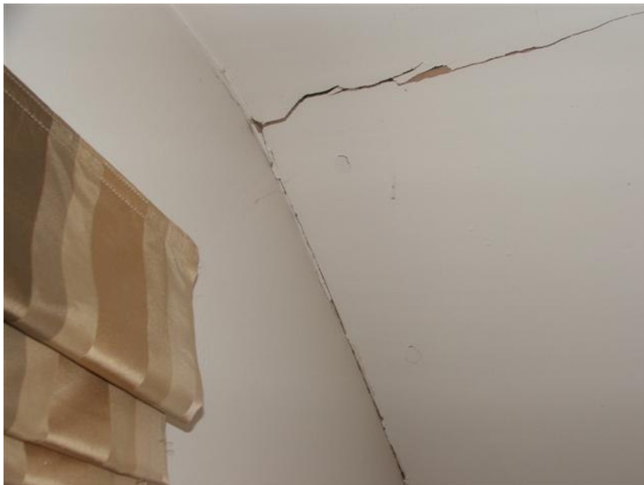
Photo 10: Showing the crack at the ceiling of the walk in wardrobe.
