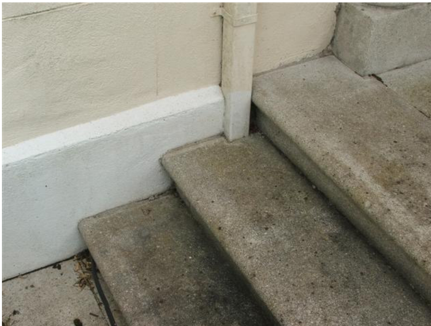
Photo 6: Showing down pipe with no identifiable means of discharging the surface water.
