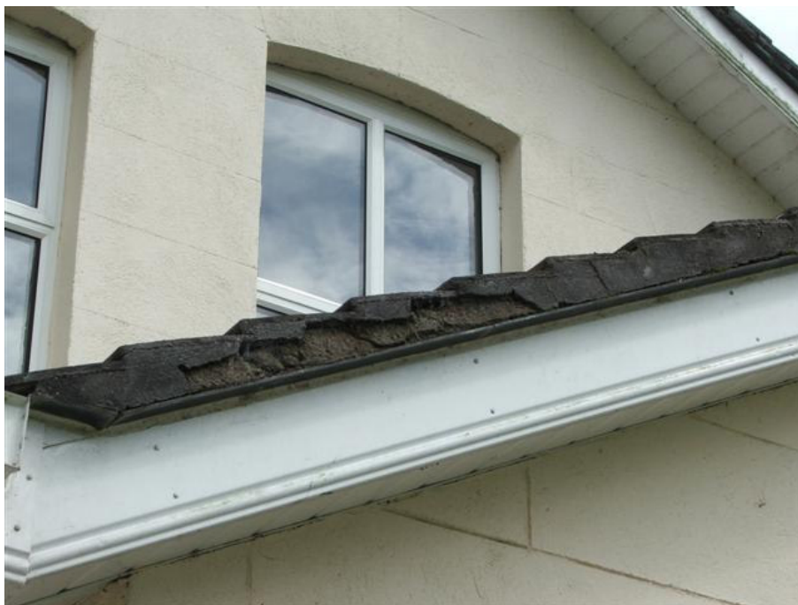
Photo 1: Showing bedding mortar missing from eaves of porch.
