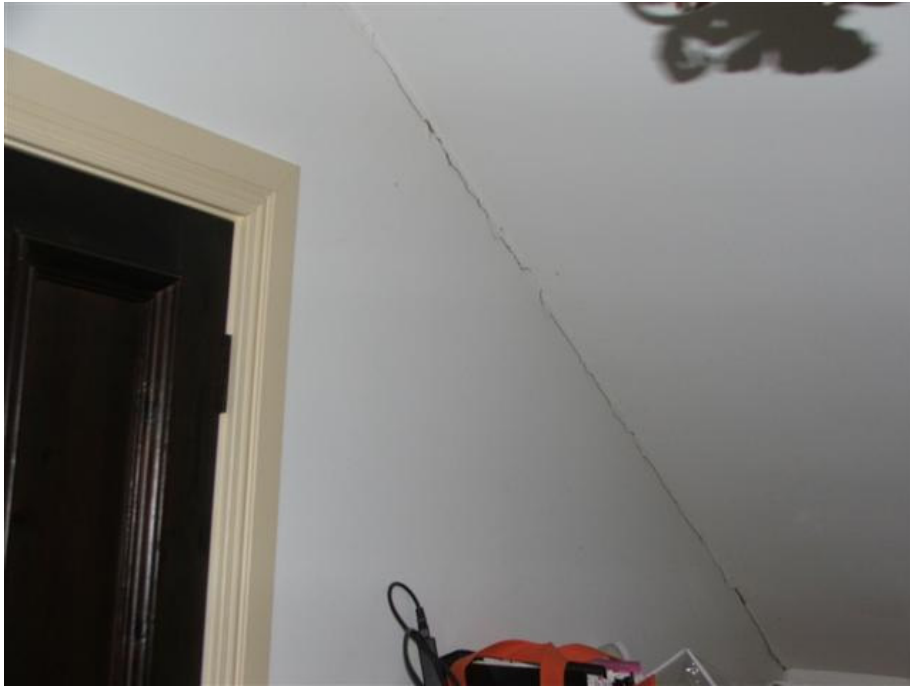
Photo 9: Showing the crack at the ceiling of the walk in wardrobe.
